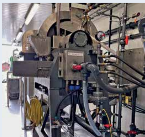
Fig 1. Magnetic separator in the pilot plant
